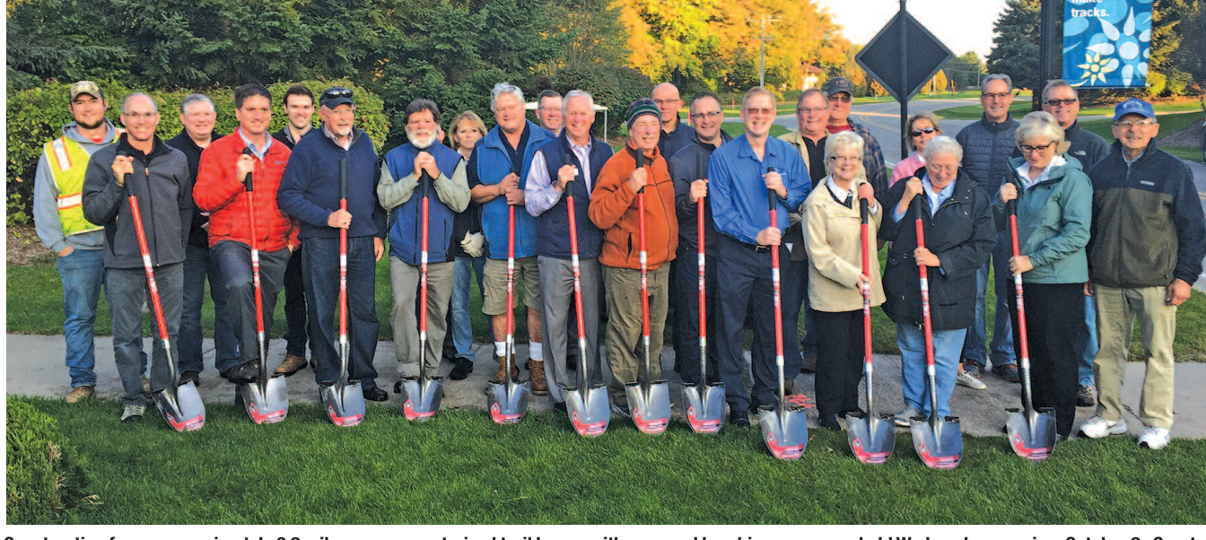
Construction for an approximately 6.2 mile new non-motorized trail began with a ground breaking ceremony held Wednesday morning, October 2. Courtesy photo
